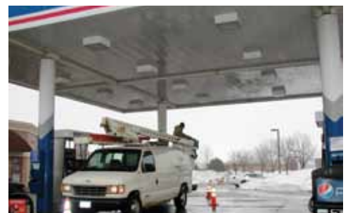
An electrician from Medina Electric prepares to install the CFL assembly kit into the existing fixtures on the canopy at Marathon Convenience Store in Apple Valley.
